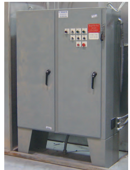
Thermal oven control panel.
