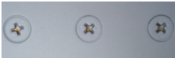
Close up view of painted fastener heads. Coatings must be capable of fully protecting the fastener as well as the interface between the fastener and skin to help reduce galvanic induced corrosion.
