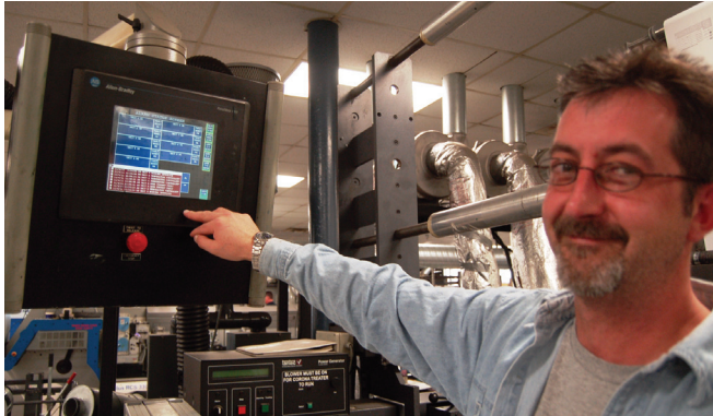
Centralized UV lamp controls make it easy for technicians to quickly fine-tune the output of each curing station to achieve the perfect results.
