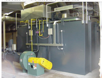
RTO scrubber system.
