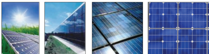
Example of installed solar panels.
